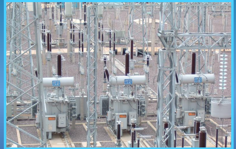
Grid Reliability and Modernization
