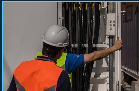
COMMISSIONING AND INTEGRATION OF MICROGRID ENERGY SOURCES
