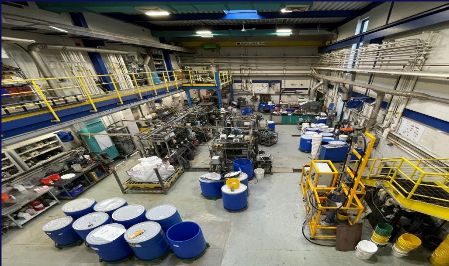
| Mineral Processing Pilot Plant at Sheridan Park
