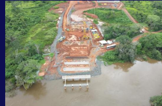
Bacaba: Execution of the bridge civil works; it will connect Bacaba to Sossego's Mill Complex
