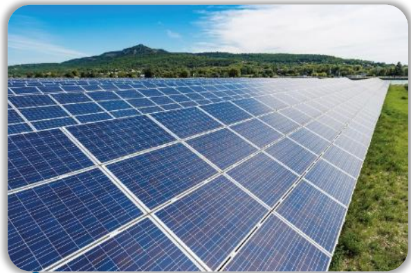
System installed by EGSD.
